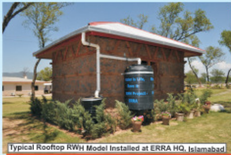
Typical Rooftop RWH Model Installed at ERRA HQ, Islamabad
